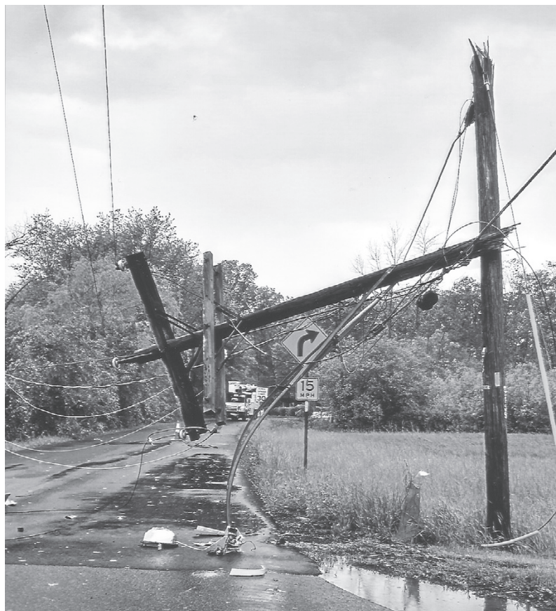
Pictured is one of several broken power poles on Grand Island following a stormy Tuesday night into Wednesday morning. This one is located on West Oakfield near Beaver Island State Park. (Photo Garnet "Sam" Pauley Larry Austin)
